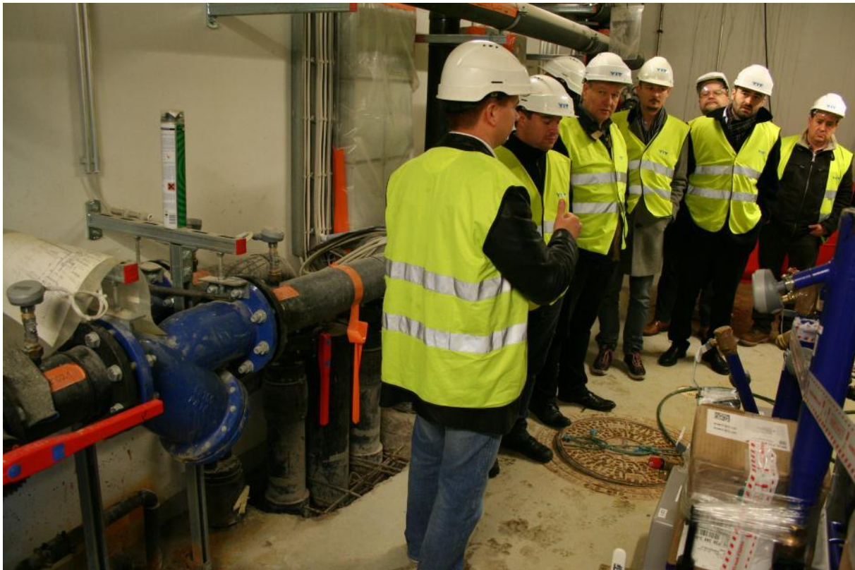
Figure 24 . EEPOS team and the some pipes and valves of the seawater cooling system
