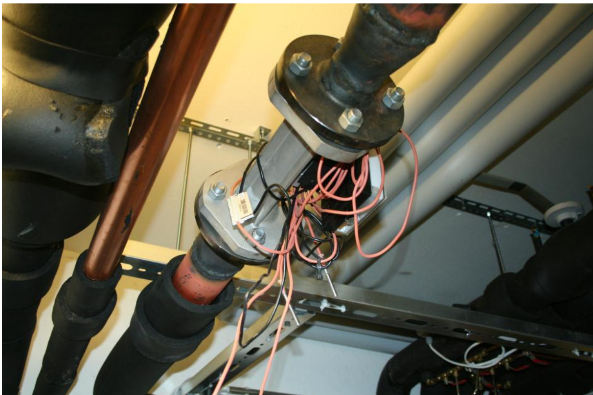
Figure 25 . Huge energy meters installed for seawater flow and related energy metering
