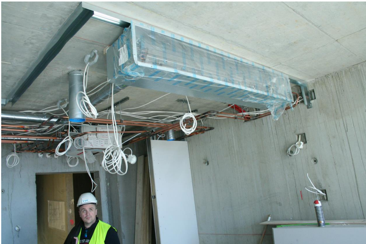
Figure 26 . Chilled beam for cooling the apartment (picture taken at construction phase)
